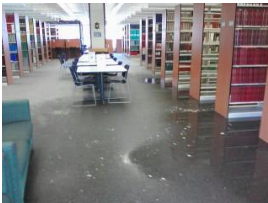
Image 3. Health Science Library Shelving Units flooded.
